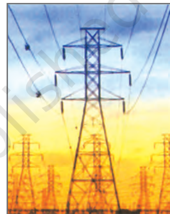
Fig. 3.7: National Power Grid to supply Electricity
