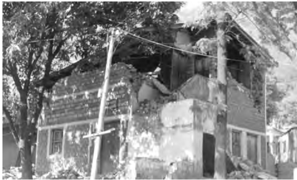
Figure 7.1 : A Damaged Building Due to an Earthquake
